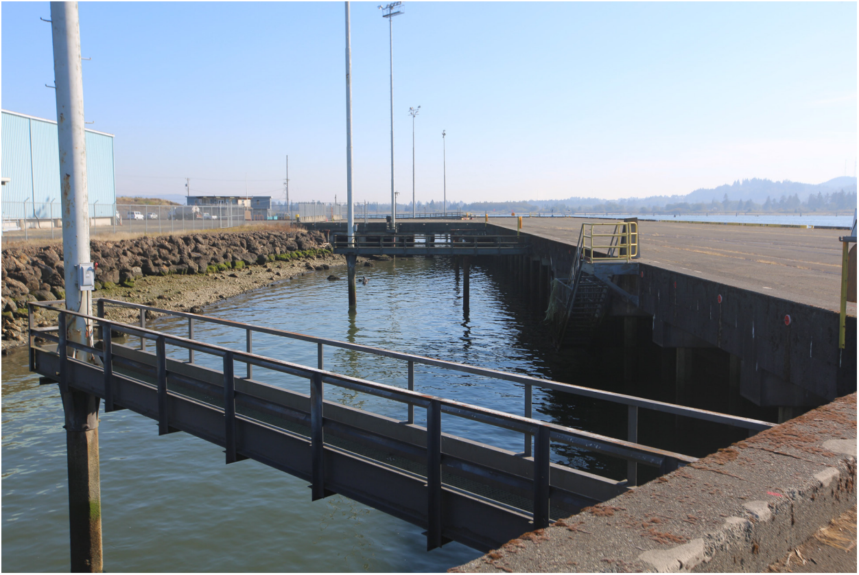
Photograph 4 Existing Terminal 4 Dock and Shoreline of Grays Harbor. Photograph Taken Facing East, 10/14/2022.
